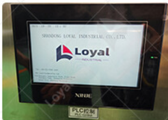
1. PLC control system
